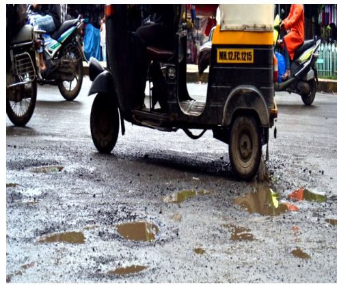
Fig. 3. Potholes and damaged roads
