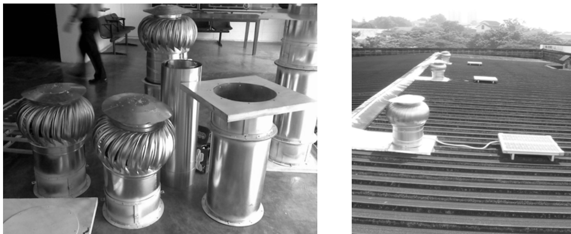
Fig. 2. Configuration of the HTV (a) before installation (b) three complete sets of the HTV installed on the roof
